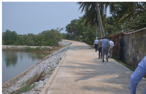
Reinforced embankment in Tam Ky District to protect agricultural land and allow resettlement. The community has also reforested it with mangroves to protect the dyke.
