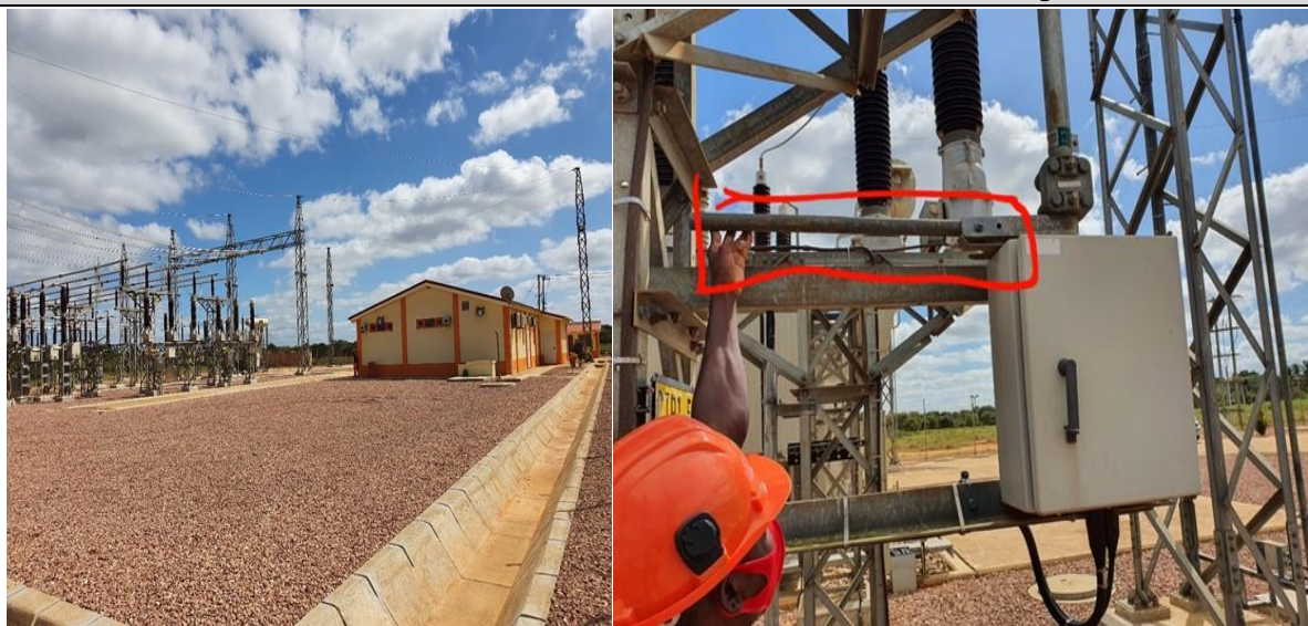
Massinga substation; Switch placed too high, making it difficult to manoeuvre
