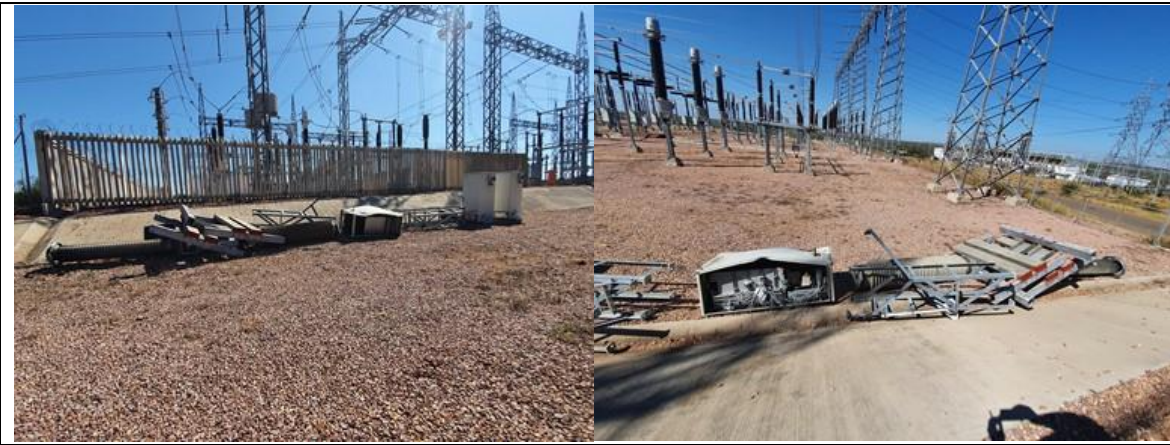
Burnt out Circuit Breaker (disjuntor) Unit
