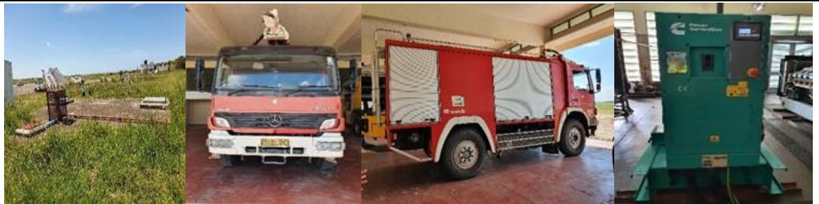
From left to the right: Water reservoir and water pump, fire fighting vehicle (Rosenbauer) and power generator.
