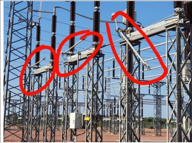
Earth switches not aligned
