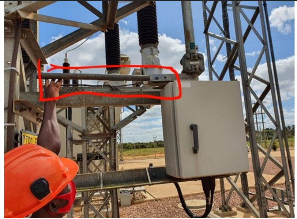
Switch placed higher, making it difficult to manoeuvre
