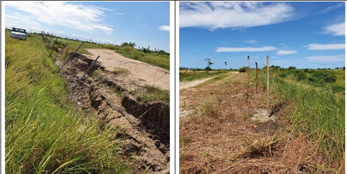
Field visit photos - fencing damaged by gully erosion created by cyclones (left) and ADM efforts to replace damaged fencing (right).
