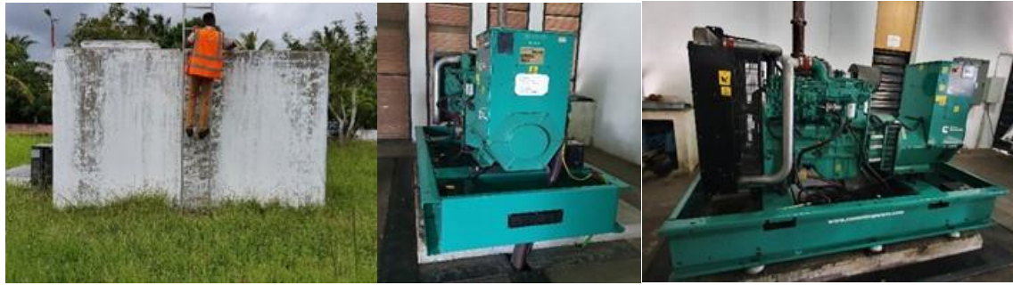
From the left to the right: Water reservoir (left) and the emergency generator (right)
