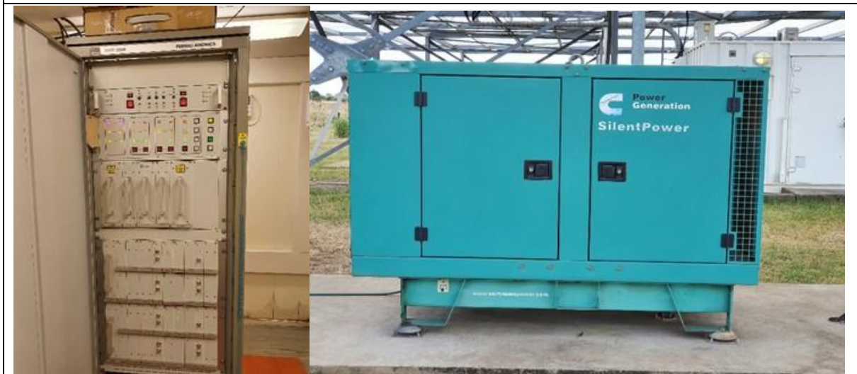
From left to right: DME (left) and a 22KVA power generator installed at the DVOR centre
