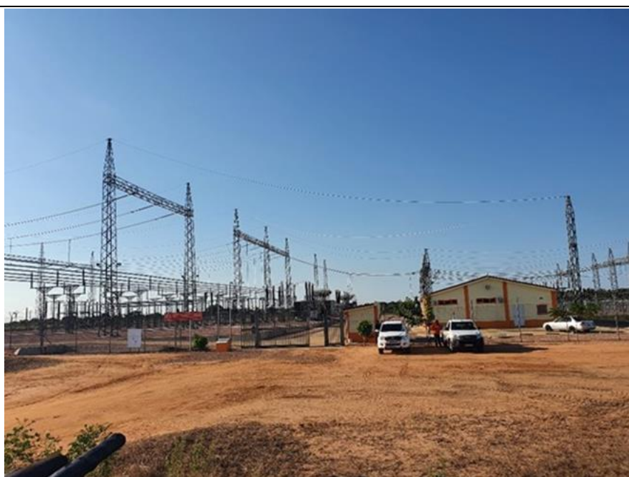
Zimbene Substation (Macia)
