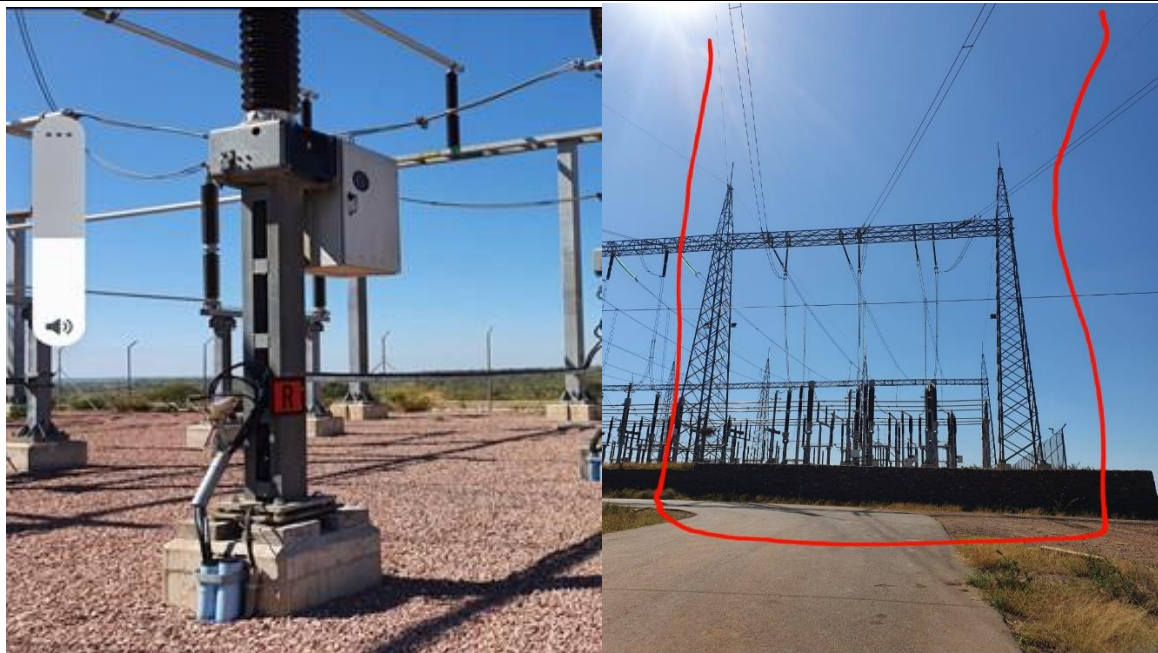
Circuit Breaker Replaced (left) Unit (BL5) constructed with Danida funding (right) leading to Zimbene
