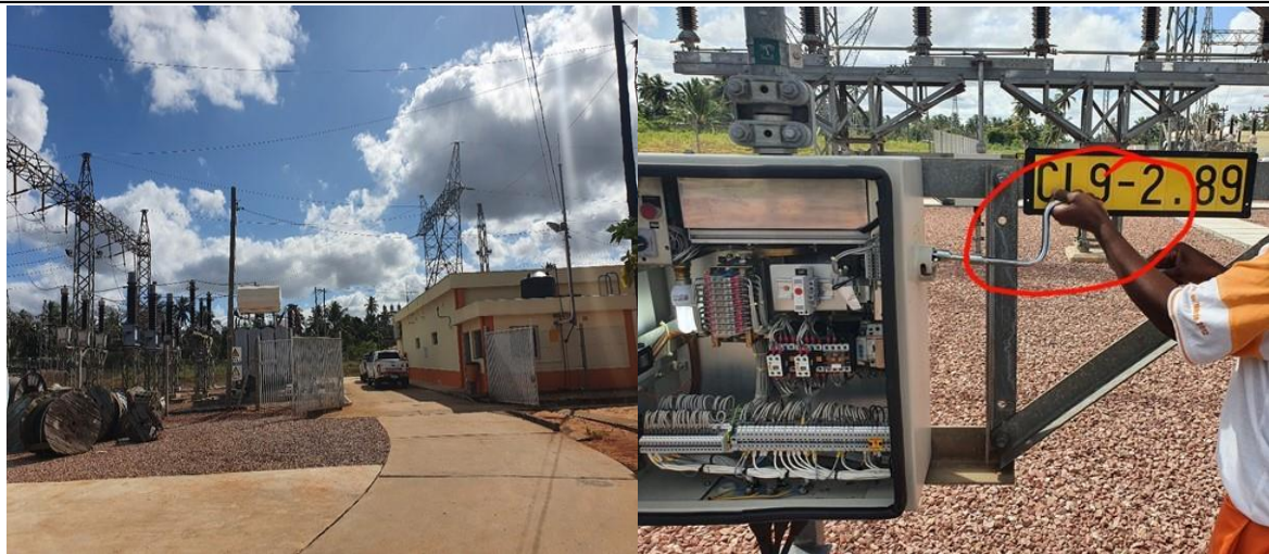
Lindela Substation; Switch placed where it is difficult to manoeuvre
