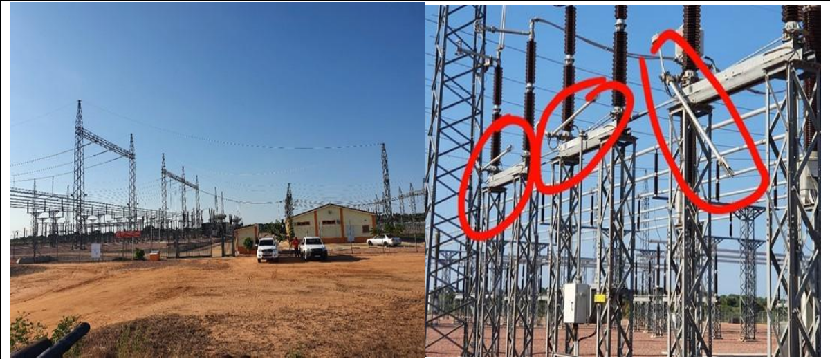
Zimbene Substation (Macia)
