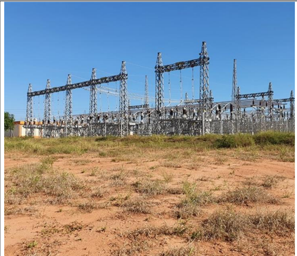
The four 66Kv exit lines of Maputo 275
