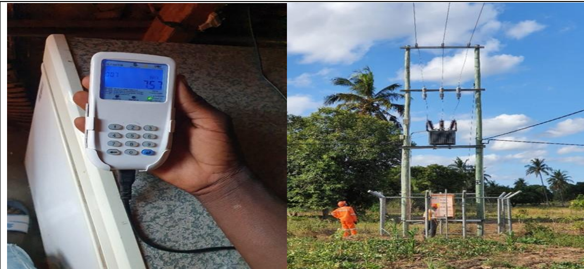
A split meter (left) and a transformer (right) in Homoine district
