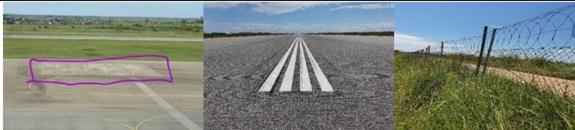
From left to right: Rehabilitated stand (left), airstrip (centre) and fencing (right)
