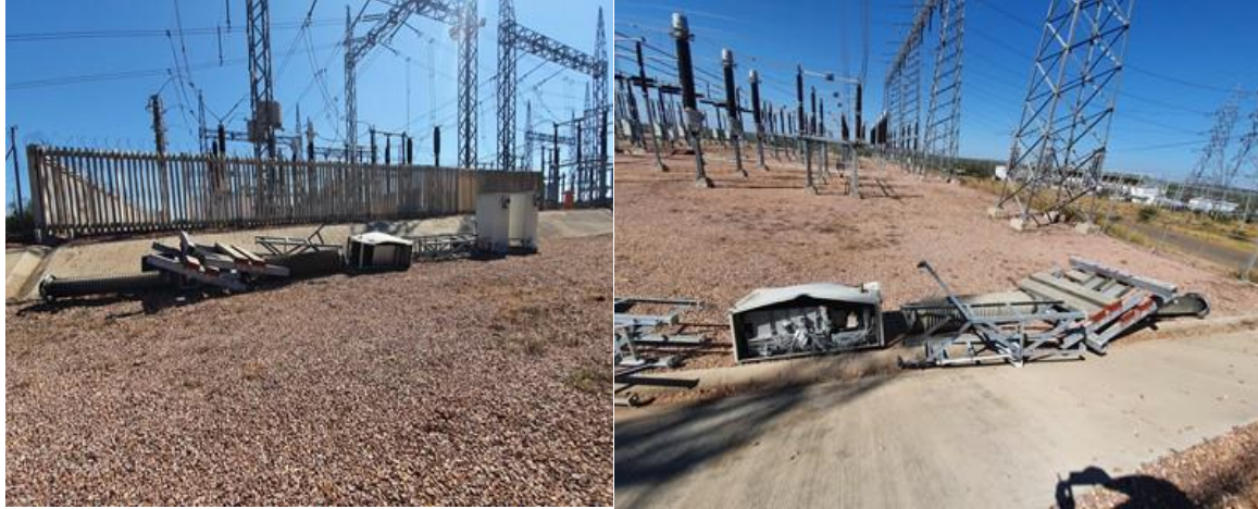
Burnt out circuit Breaker (disruptor) Unit 123
