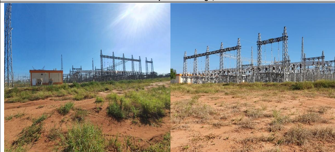
Maputo 275 Substation; The four 66Kv exit lines of Maputo 275
