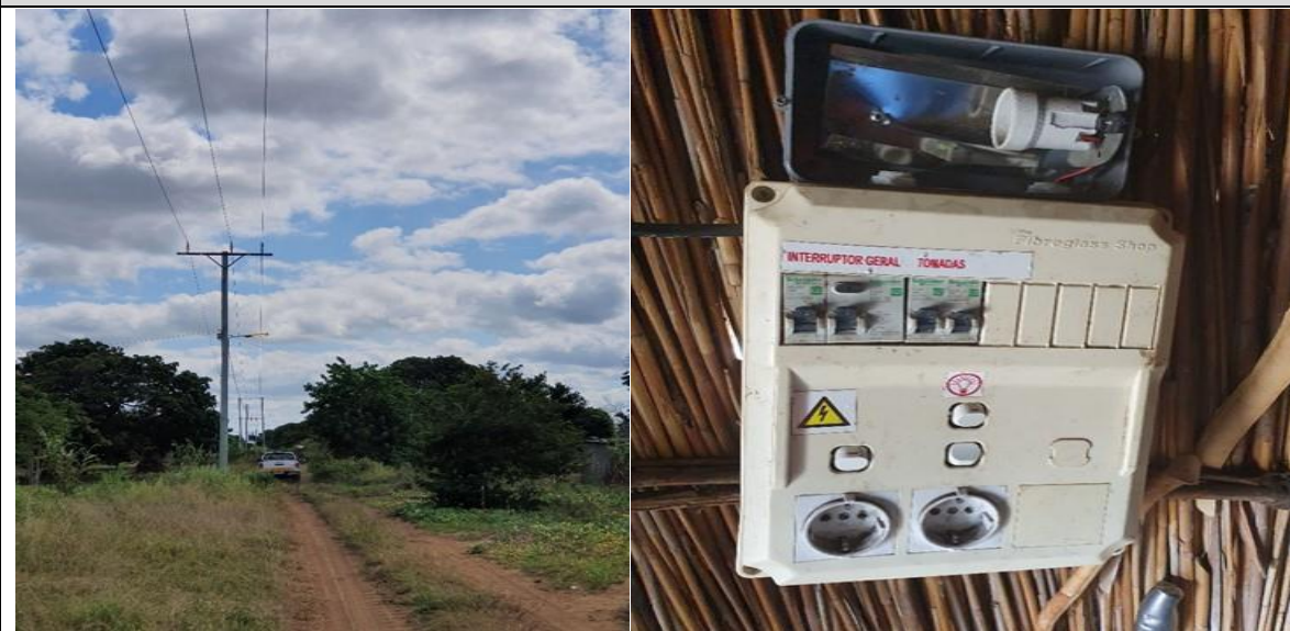
Rural electrification in Muxaxane - Chibuto (Power line on the left and integrated meter on the right)
