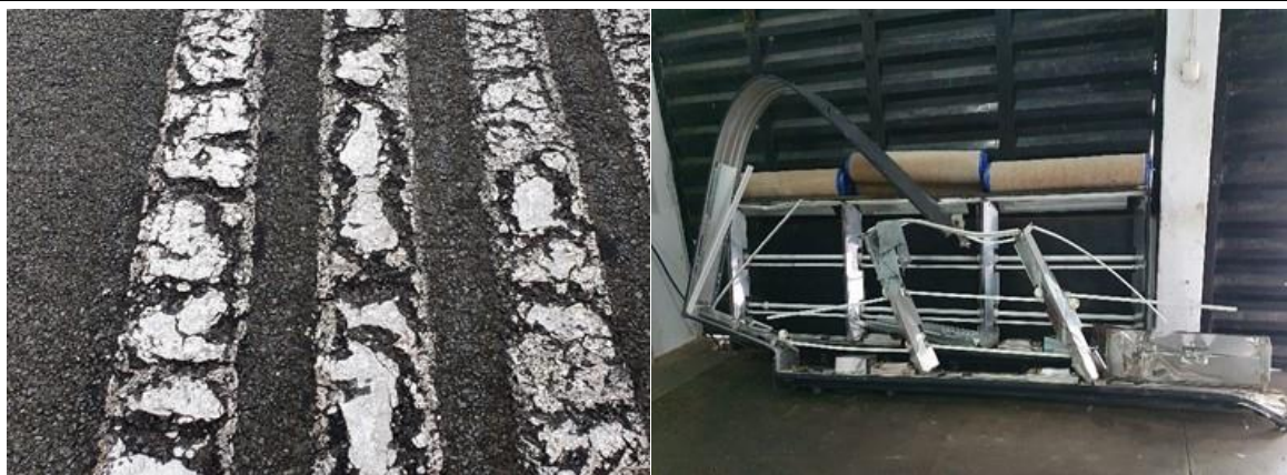
From left to right: parts of the airstrip degraded by the paint (left) and vertical sign damaged by the plane that ran out of the airstrip in 2020.
