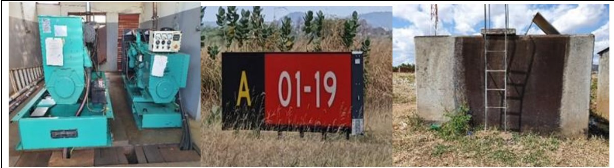
Field visit photographs - from left to right: Two power generators (left), water reservoir (centre) and vertical signal (right)
