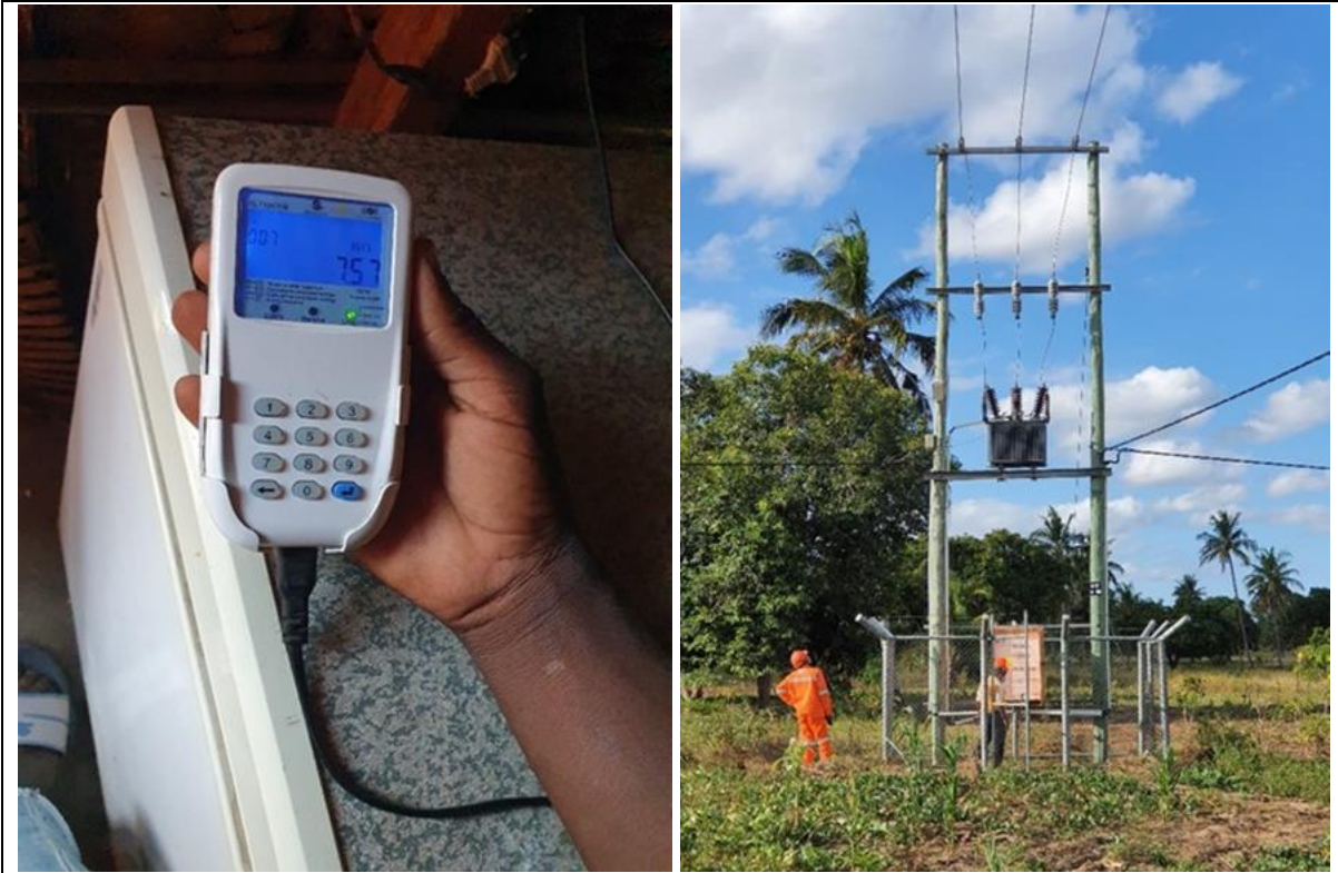
A split meter (left) and a transformer (right) in Homoine district
